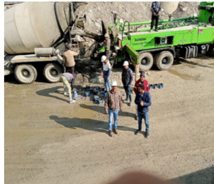
Construction of 4 Laning of part of Ramban to Banihal of NH-1A (NH44)
